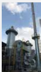
Air pollution control system
